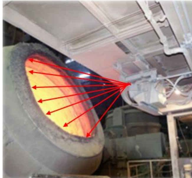
Figure 9: Laser scanner measures on the internal surface of the ladle from the outside the steel ladle
