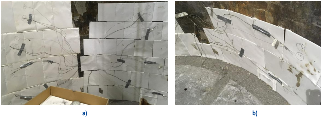
Figure 7: Installation of thermocouples on steel ladle lining: a) front view; b) top view.
